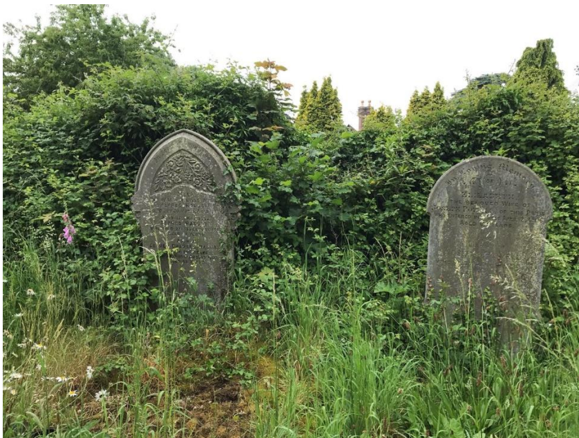
Western wall – the area from the grave stones back to the wall (1.5 – 2ms wide) is overgrown with brambles and ivy.
